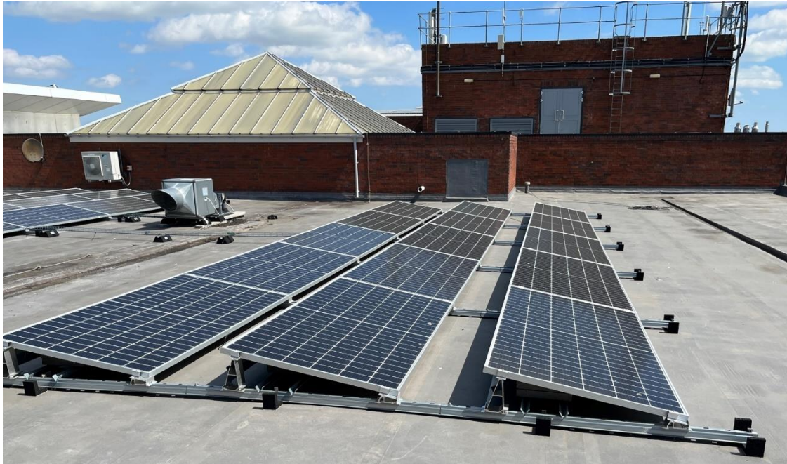
Figure 2: Solar panels on the rooftop of the Louisa Leisure Centre in Stanley
