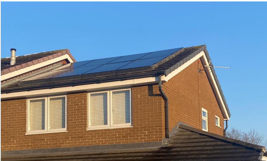
Figure 1: Solar panels on a residential property.
